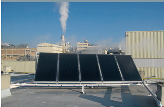
Pilot projects: In Spain, we have installed small-scale solar thermal systems at our sites in Seville and in Montornès (photo). These systems use the heat from solar radiation to provide hot water for the sites.
